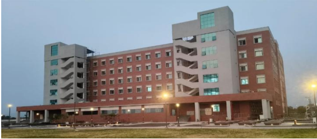
Construction of Shri Ramchandra Institute of Medical Sciences (SRIMS) College - Nursing College Building classroom in Aurangabad
